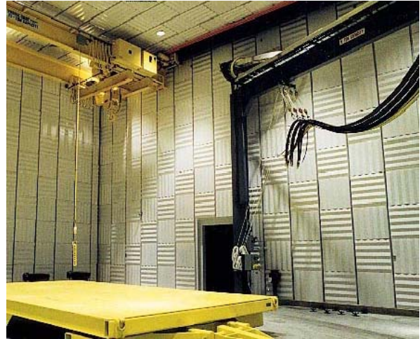
Fig. 8 Large Free Field Chamber, York International PA. U.S.A.
